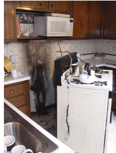
The Nott's fire-damaged home survived, thanks to a quick response.
